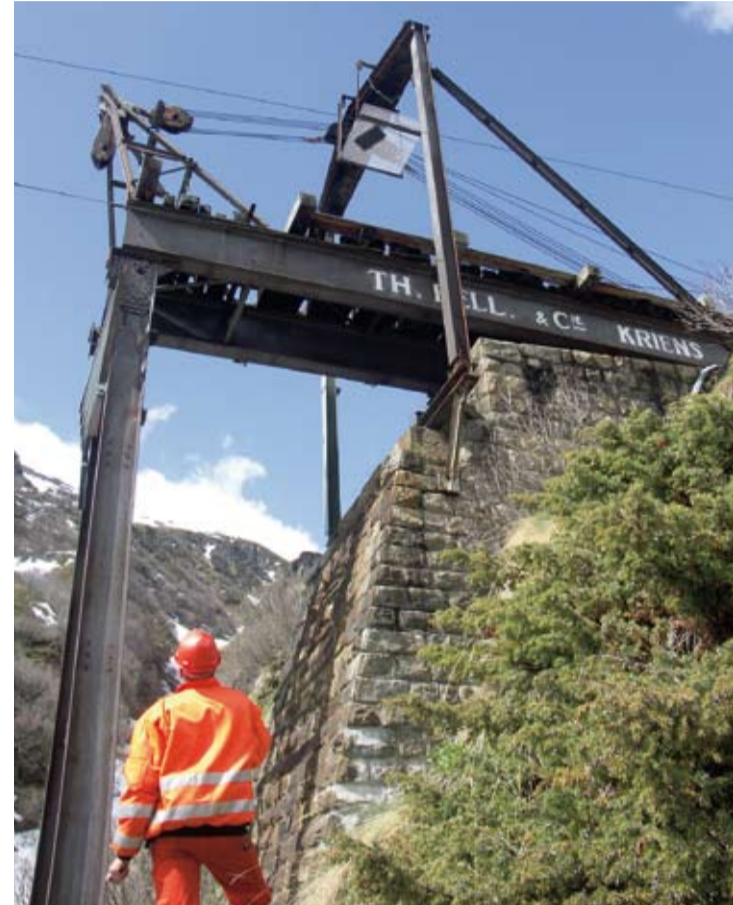
Folded down middle section of the Steffenbach bridge.
